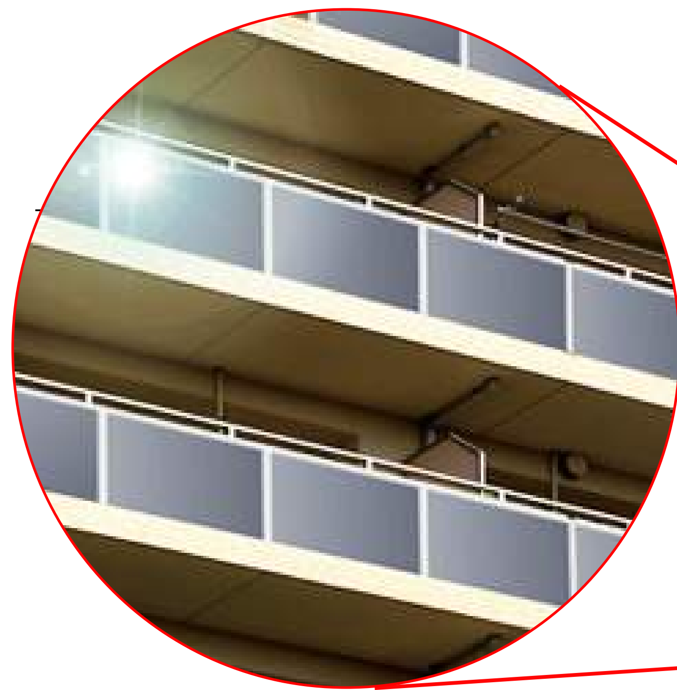
Transparent solar panel on railing
